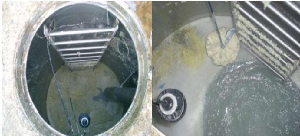
Grease Buildup In Wet Well Before Treatment With EnviroDEFENSE® FOG Degradar
